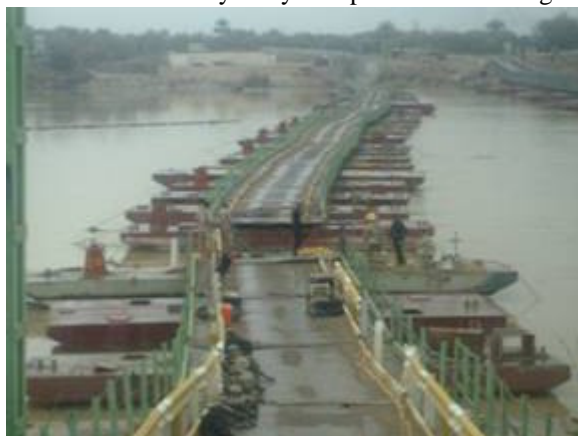
This is the bridge that we repaired, note the big hole.
