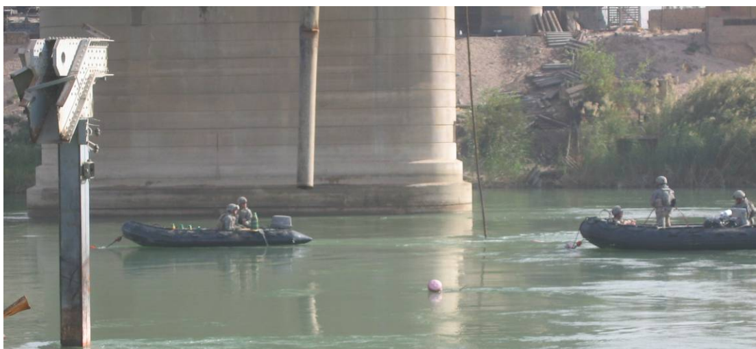
Members of 7 th Dive Lowering Shape Charges to Diver Located on Submerged Bridge
